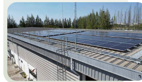
Installed a solar rooftop at the waste sorting facility with a total installed capacity of 52 kWp
