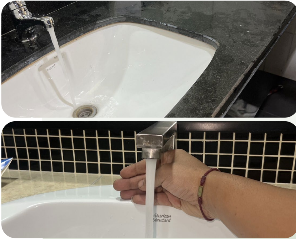
Replace conventional water taps with sensor-activated faucets to conserve water in male and female restrooms on Floors 2-4 of the AMATA Service Center building
